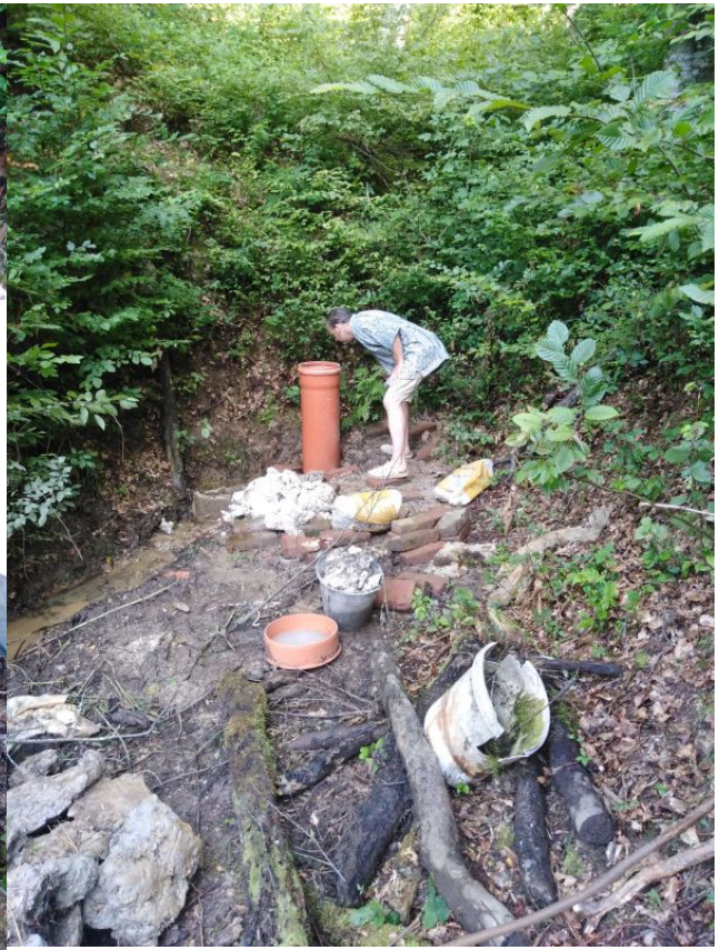
now with a new pipe and lid
